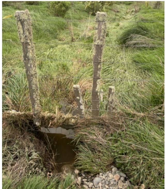
Figure 11. Outlets should direct water to a filtration area and not bare soil.
